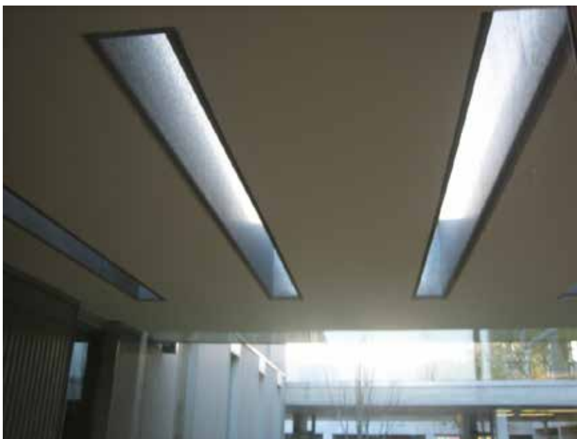
Gaps in the entrance of the building
