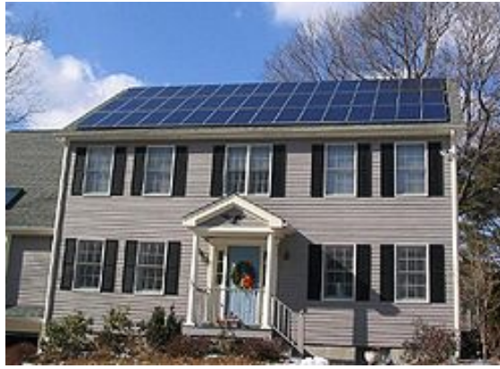
Photovoltaic solar panels on a house roof
