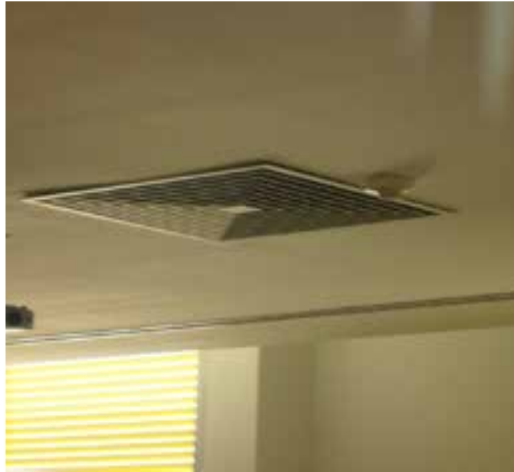
Ventilation on the roof (50*50 cm)
