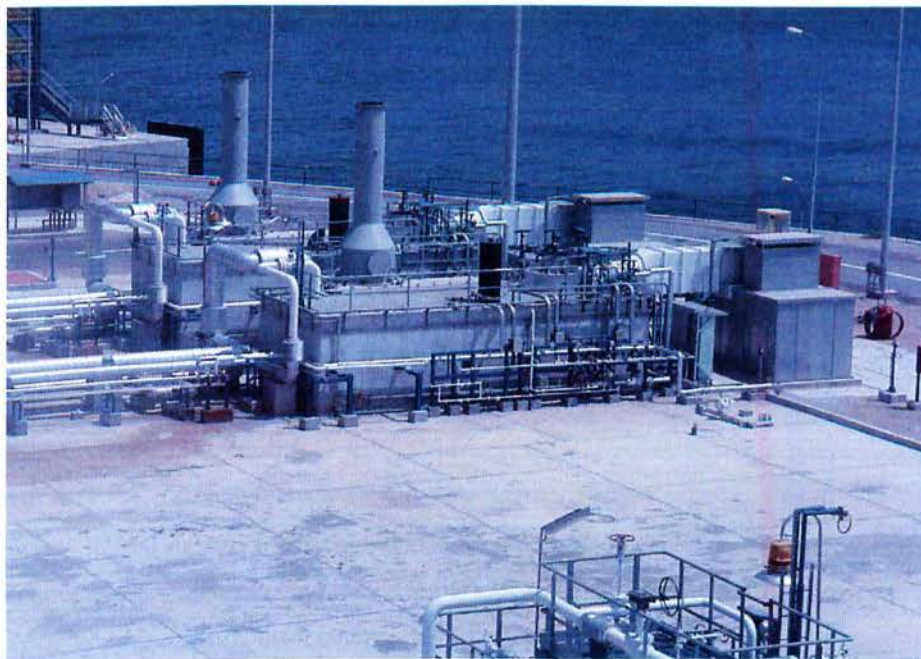
Submerged Combustion Vaporiser . SCV
